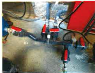
Figure 5 – Mobile System Piping
