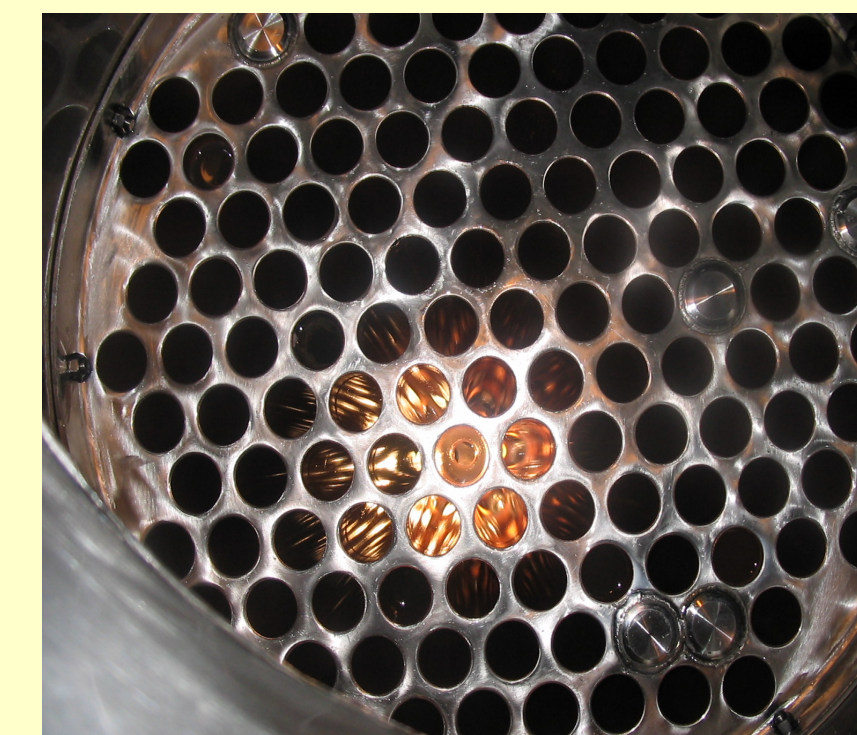
Figure 6 Clean calandria tubes after caustic/peroxide wash
