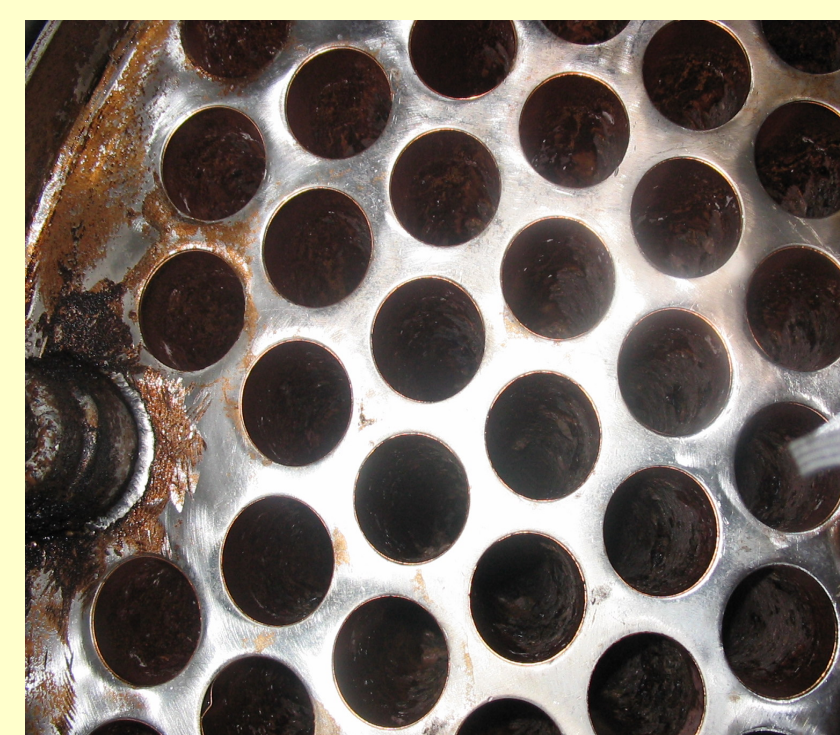
Figure 5 Calandria tubes with deposits after caustic only wash
