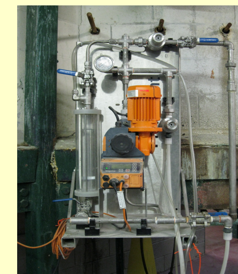
Figure 2 Picture of Peroxide dosing Equipment
